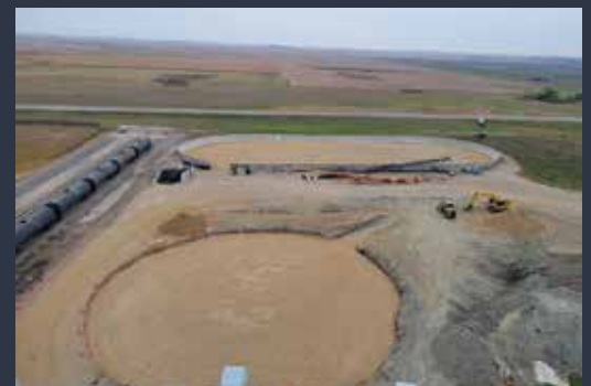
Progress continues on the new 1.2MM bushel corn bin in Mina. Once complete, we will have 4.85MM bushels of storage onsite. This project should be completed just in time for next year’s harvest.
